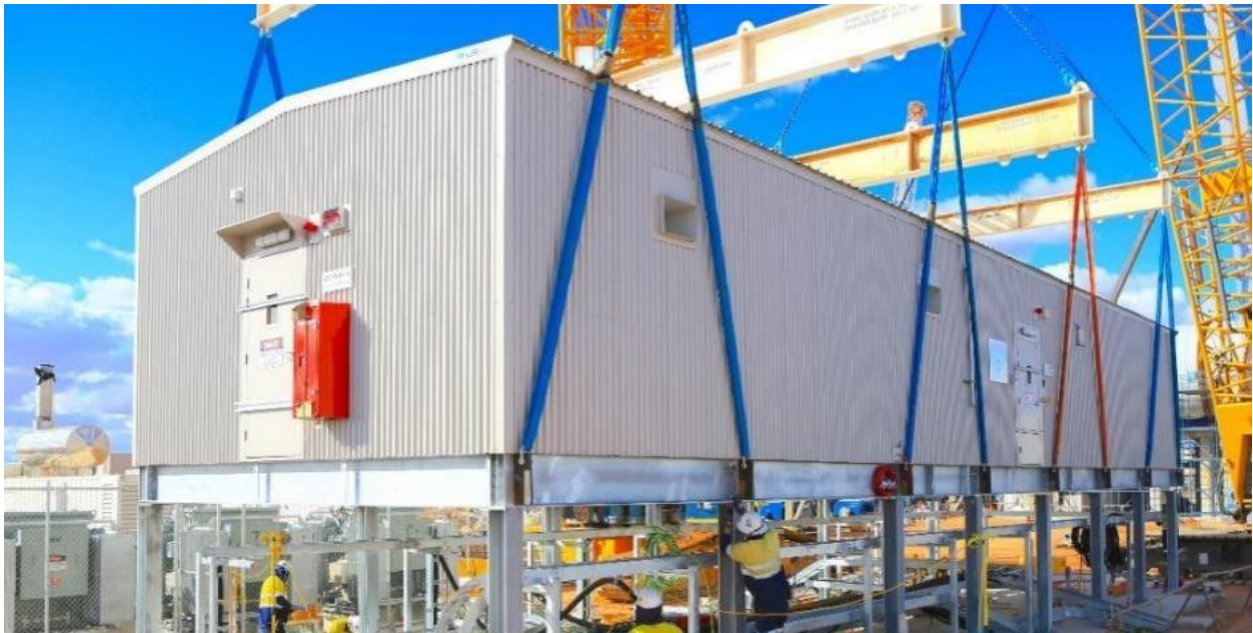
Figure 3 Control Room Example
